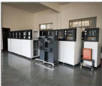
Control Cabinet Lab
